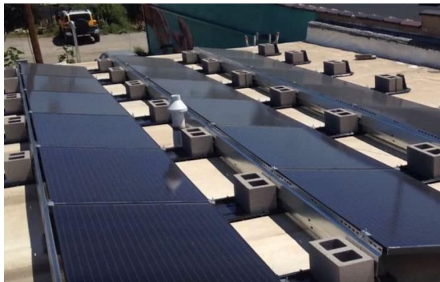
Laramie's Downtown Clinic's 25-panel solar array offsets 98% of the clinic's energy usage. The project also includes Wyoming's first Blue Sky battery storage system, which will keep medical supplies, such as vaccines, properly stored during an emergency. A $33,675 grant from the Rocky Mountain Power Blue Sky Program made it possible.
